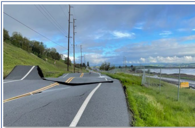
Figure 5 - Highway 1 Storm Damage
